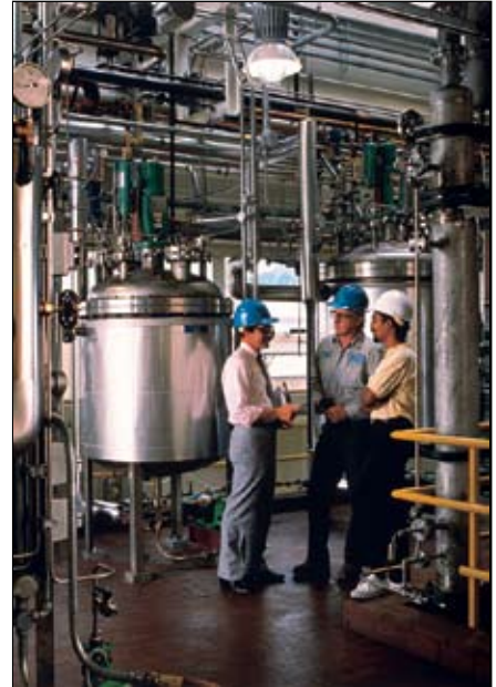
Stainless Steel FRLs in this pharmaceutical plant are used for valve protection and lubrication at point of use applications.
